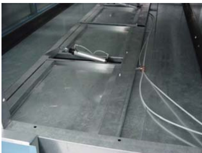
BYPASS DAMPER CLOSED (SPRAYING PHASE )
