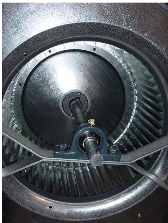
TRANSMISSION SHAFT BEARING AND WHEEL
