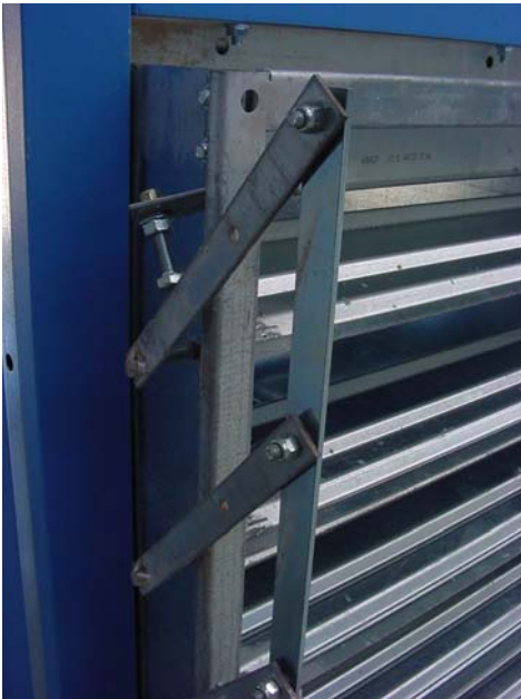
SETTING SCREW TO KEEP THE ABSORPTION OF THE INTAKE MOTORS WITHIN THE NOMINAL VALUE
